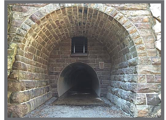
Renovation of the Poe Paddy Tunnel highlights the cooperative venture of State agencies, commissions and associations to meet the safety needs of the public while preserving and protecting a unique aspect of its environment.
