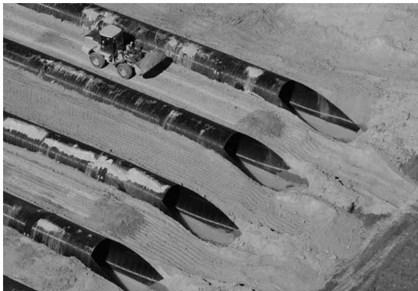
Figure 26. Compacted side fill should be completed on both sides of structure before fill is “carried over” for construction traffic.
