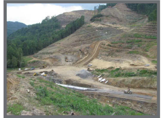
Wyco Hollow at the headwaters of Allen Creek. Vantage point at final grade of the ravine crossing. An estimated three million cubic yards of fill needed to reach grade opposite side (notch to the right of upper middle-tree line).
