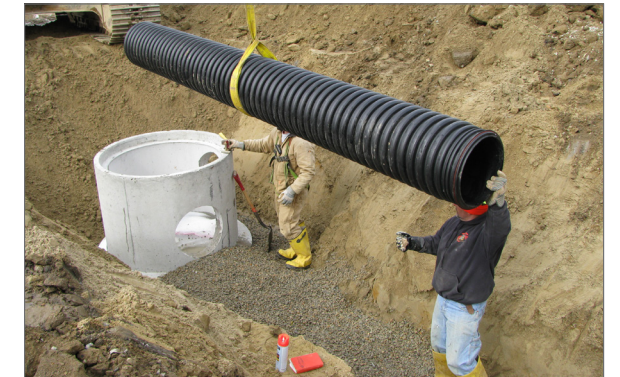
Photo illustrates single sling handling used for the smaller diameters, sloped trench walls to mitigate against the need of a trench box, and stone bedding above the trench foundation.
